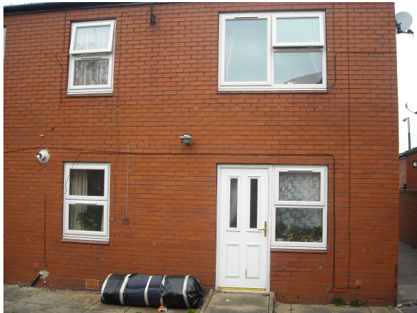
Insecured bedroom window at rear of property and Euro Profile locks that are susceptible to tampering
