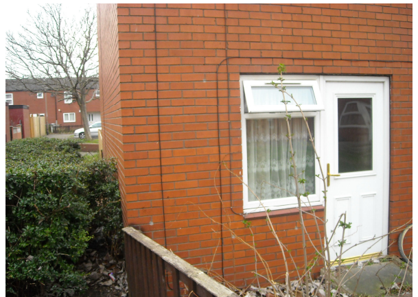
Insecured kitchen window at rear of property and Euro Profile locks that are susceptible to tampering
